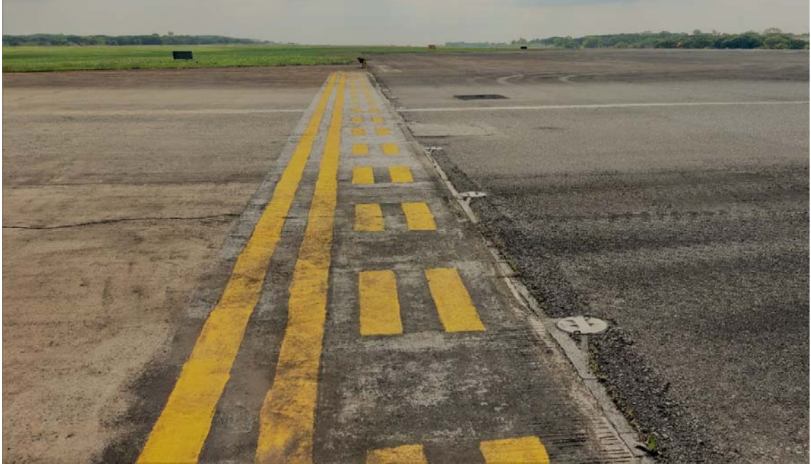
Figure (3) Runway Holding Position Marking and Stop bar Lights of Taxiway A6
